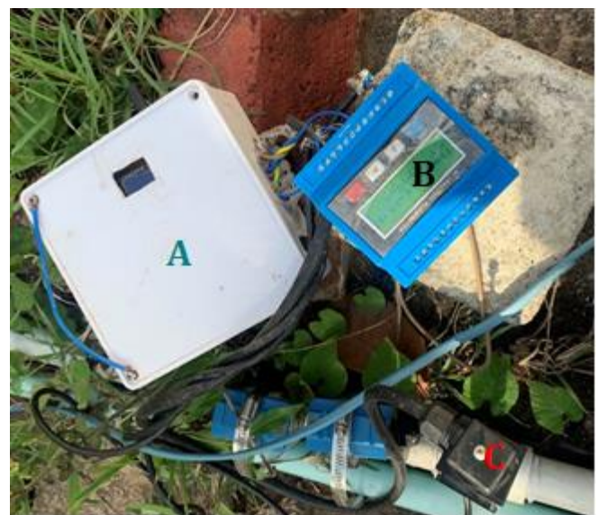
Fig. 7. A node consisting of the monitoring unit, flow sensor, and pressure sensor attached to the pipeline.
