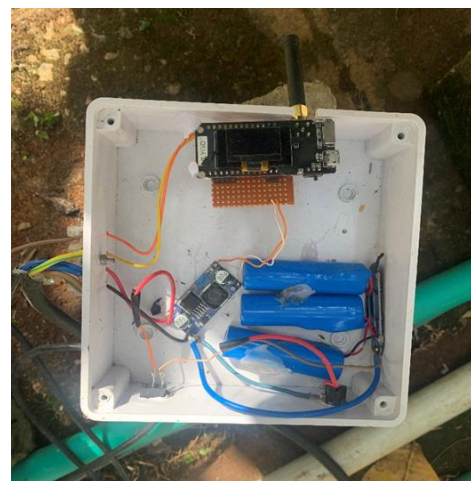
Fig. 4. Picture of the monitoring device.
